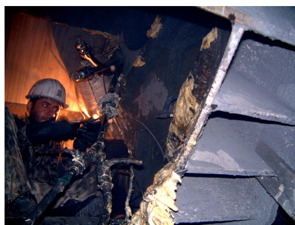
Injection of two-component polyurethane MEYCO® MP355 A3 through pipes into the void over the TBM cutterhead.
