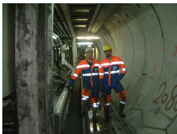
Ghomrud water tunnel during excavation. Final lining with trapezoidal pre-cast concrete segments.
