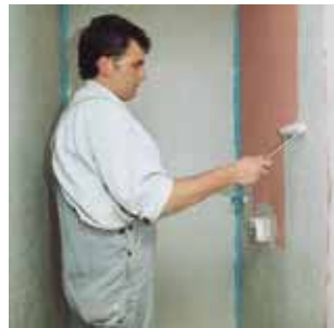
5. After an evaporation time of approx. 1 hour apply the second protective coating with PCI Lastogum (grey). The first coat of PCI Lastogum (red) should not be visible, otherwise another layer might be necessary.
