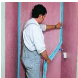
3. Fix PCI Pecitape120 with PCI Lastogum (red) in corner joints and floor/wall junctions.
